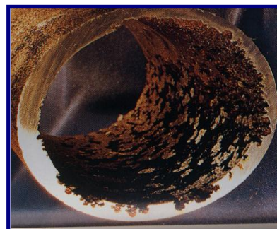
Under Deposit Corrosion View after Cleaning
